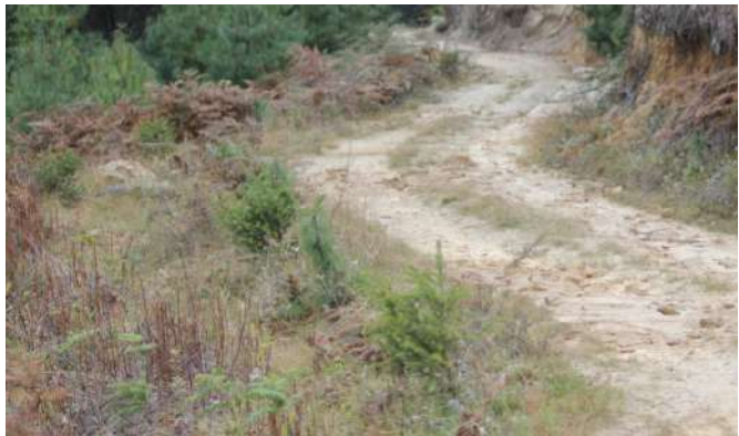
Figure 7: Lack of side drains along forest road
