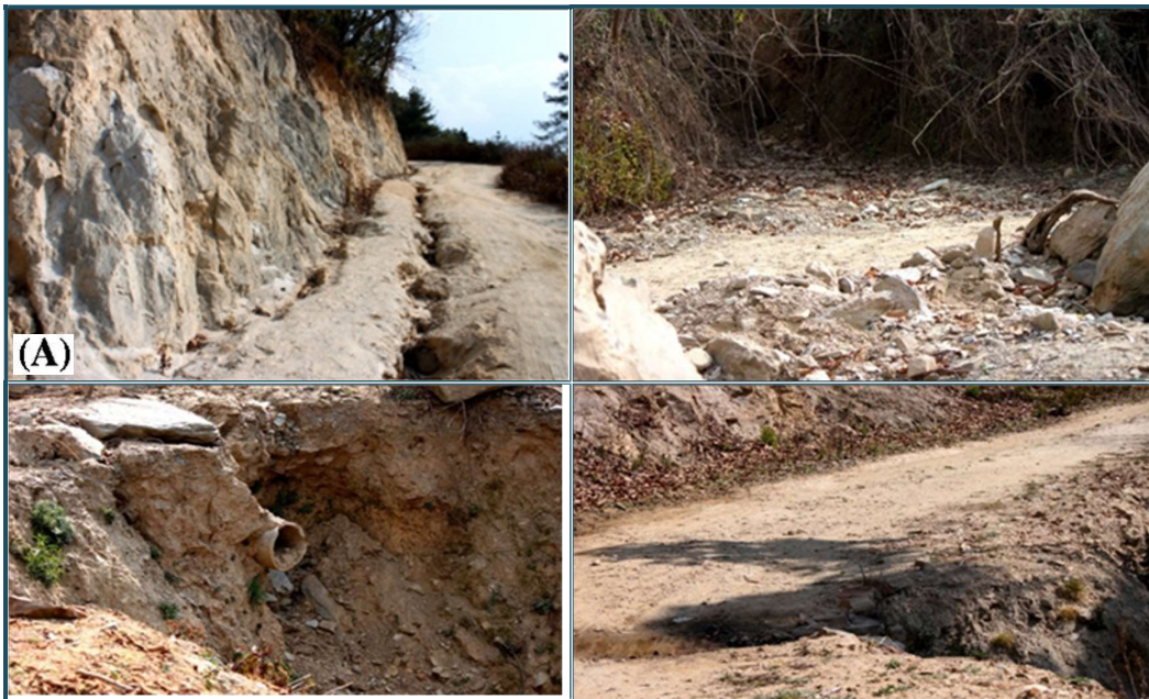
Photo 1: (A) Absence of drainage on farm roads & water channel formation. (B) Lack of catch pits on depressions & streams along farm roads. (C) Blockage of hum pipes being too small in size & also due to lack of catch pits and debris entering & blocking the hume pipe diverting water onto farm roads. (D) Gully formation on farm roads
