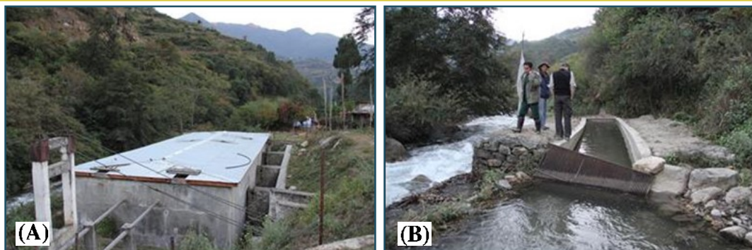
Photo 8: (A) Pretreatment tank with alum dosing & (B) Preliminary settling tank collecting debris at drinking water offtake at Rikizampa
